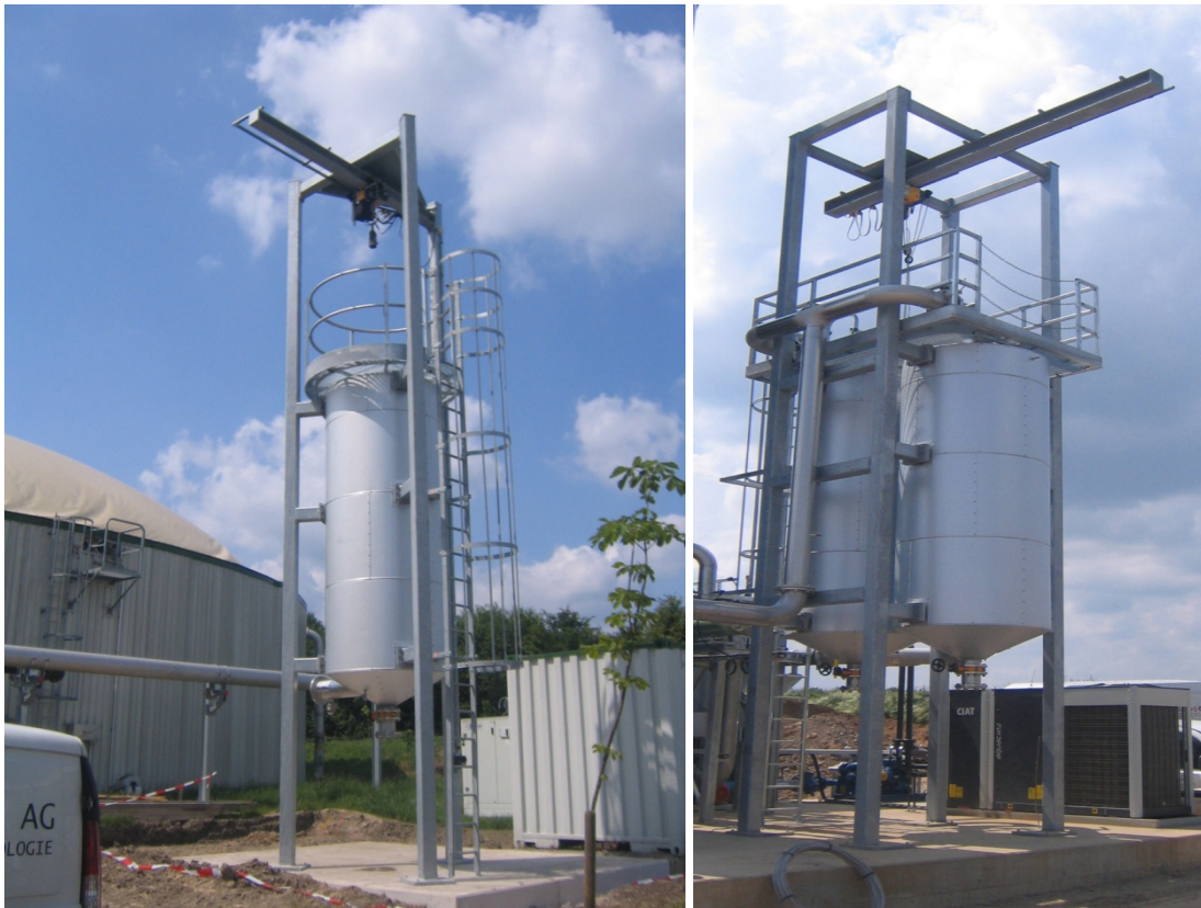
Figure 4: SILOXA FAKA 3.000 K2E and TWIN FAKA K2E gas cleaning system.
